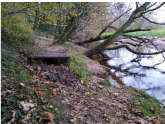
FP 22 - One of several boardwalks stood up in fresh air with mud at either end
